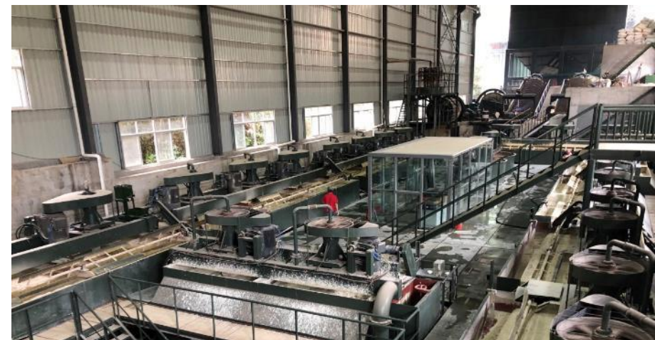
Shunchang fluorspar flotation plant, Fujian, Haojingda Industrial Co.; 600,000 tpa ore processing capacity
